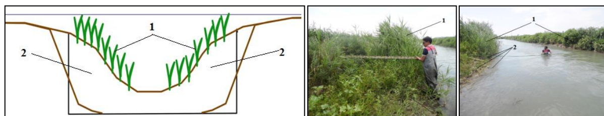
1 – overgrowing, 2 – silting (inter-farm channel K-18, Turkestan region) Figure 1 – In-situ observations of irrigation channels
